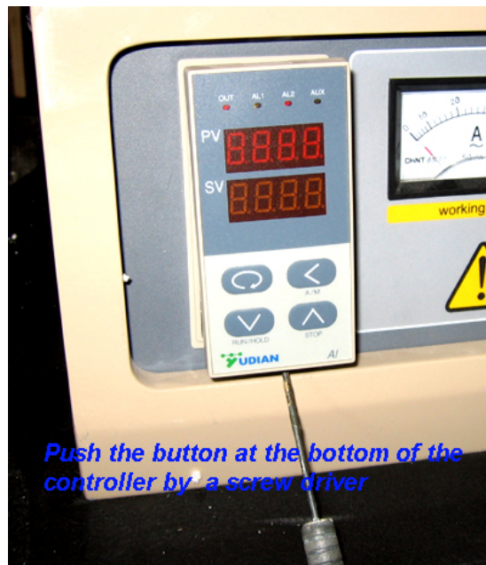
Fig.2 uninstallation of temperature controller, step 1
